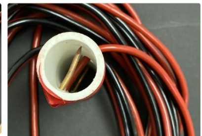
Inside ROV Power Connection
